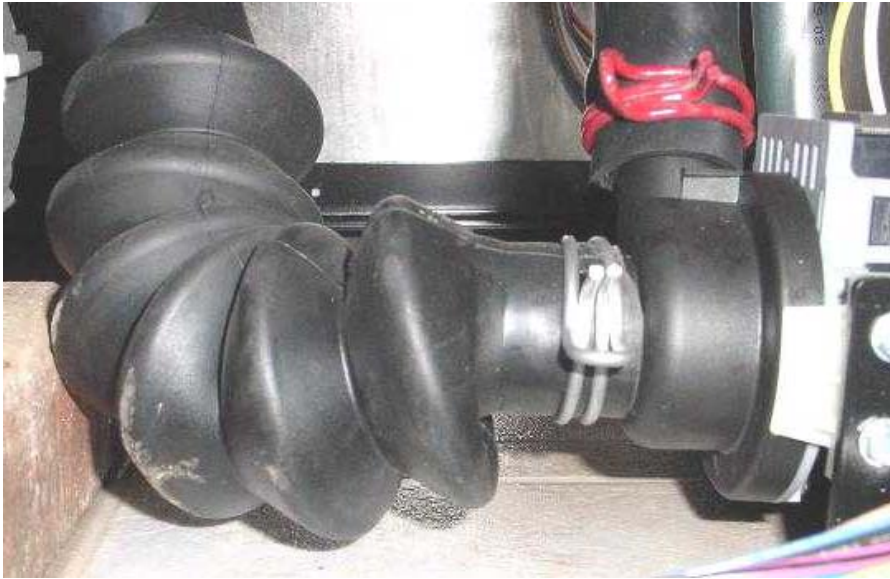
Short sump hose without hanger (notice the hose is sagging below the inlet of the pump)
